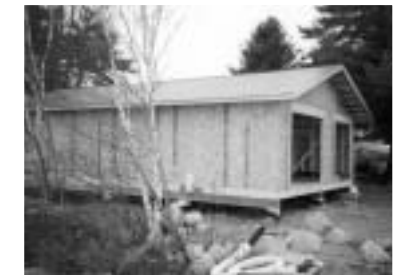
Malcolm's high school students construct the new canoe tripping room on the side of the barn.
